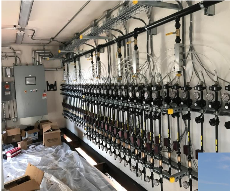
Biosparge Control Building- Interior
